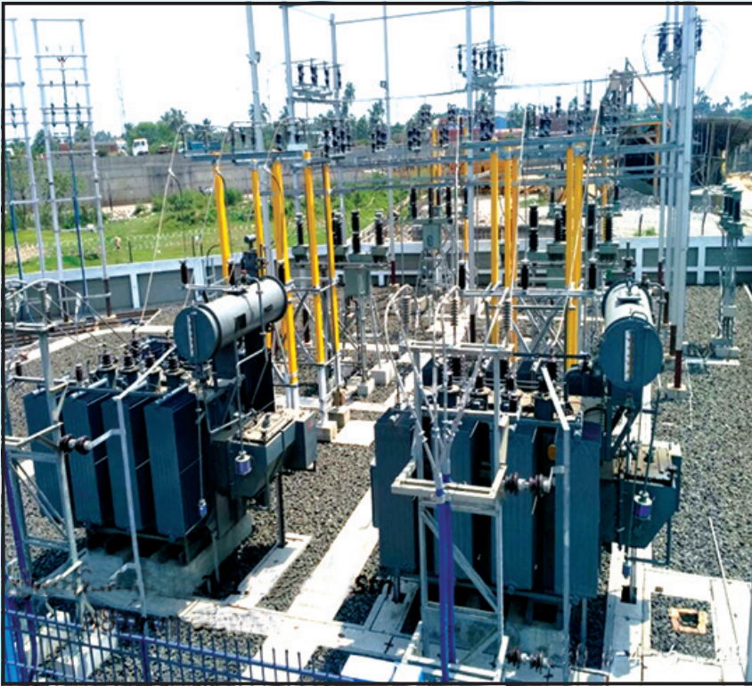
Srijan 33/11 KV Substation, Howrah District
