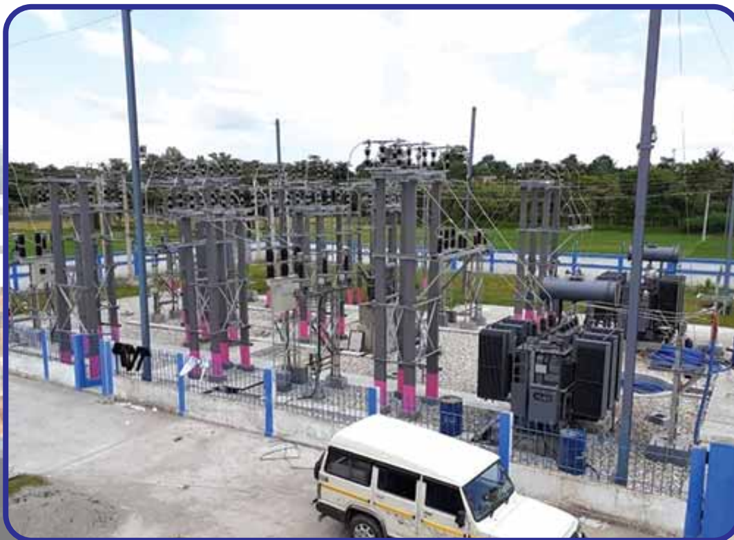
Dewanhat 33/11 kv s/s - Coochbehar District
