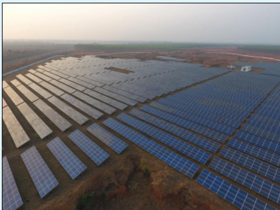
Patni Solar PV Power Plant
