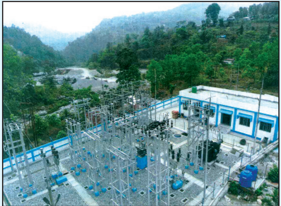
Pala 33/11 KV Substation, Kalimpong Division
