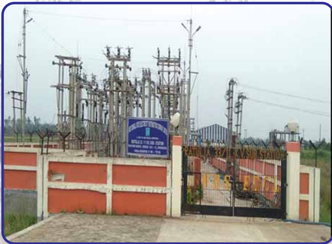
Ratulia - Purba Medinipur (Substation building)
